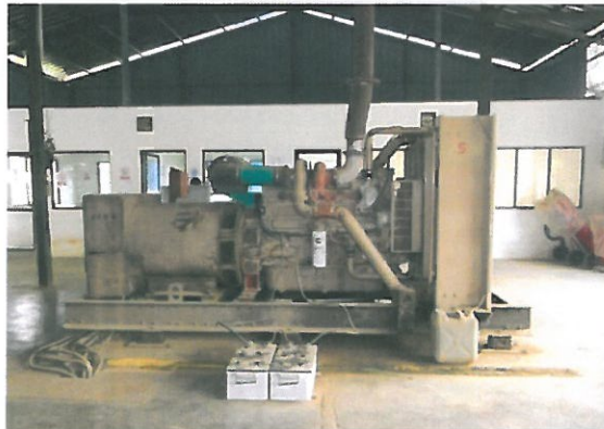
Electrical Generator (500 KVA)
