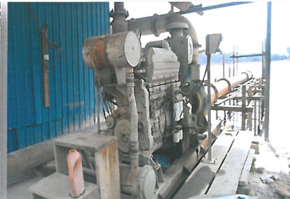
Large Diesel Engine (500 HP) for Water Pump
